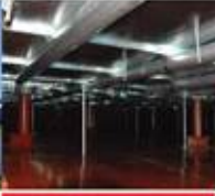
Internal Floating Roof
